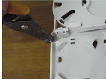
Pic7: right-routing leads in box entrance
